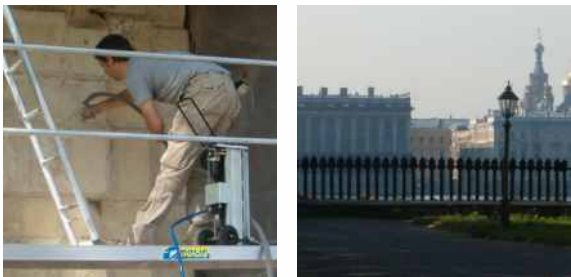
St Peter's Gate (1714) – cleaning of Kikerno (dolomite) stone, removal of finish plaster and stucco. Cleaning/sandblasting new segments of restoration stone.
